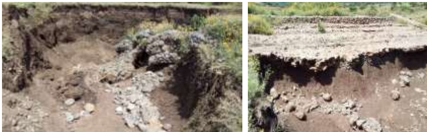
Figure 18. Check-dams demolishing and losing their physical appearance and functionality at Karamarda mountain.
